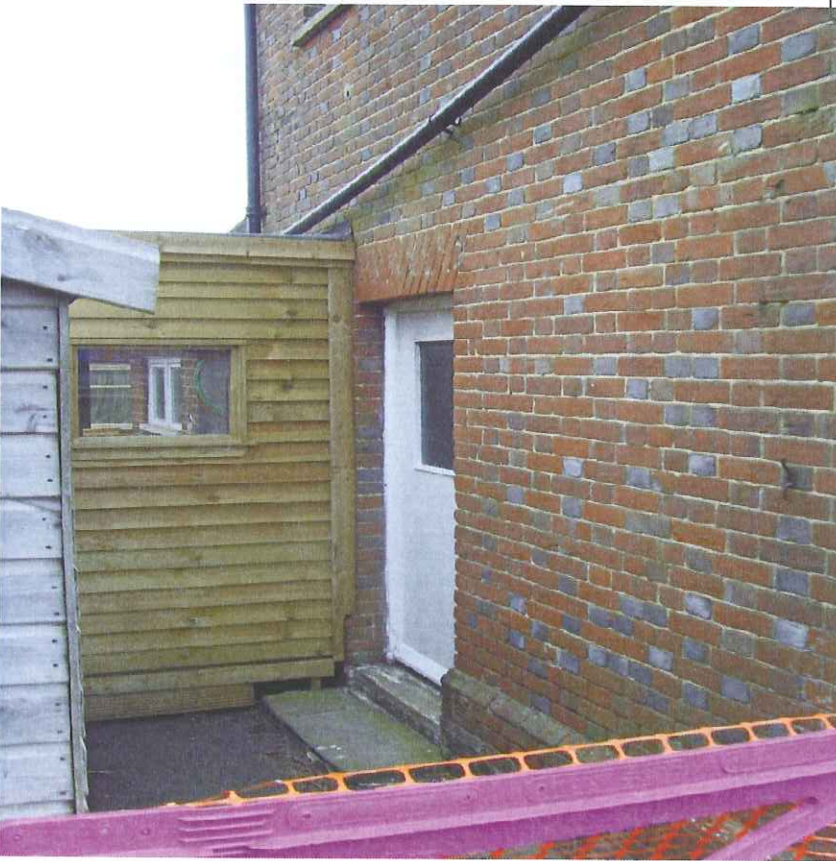
Partial view of the North Elevation, with door and frame to be removed complete and construction of 900mm height brickwork, with window to match those surrounding, fitted into the existing door opening.
