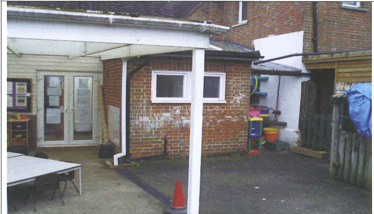
Partial view of the North Elevation, indicating area for new access ramp and replacement of double door entrance with new single door, also external recess to be in filled and polycarbonate roof replaced with new flat roof to match that adjacent.
